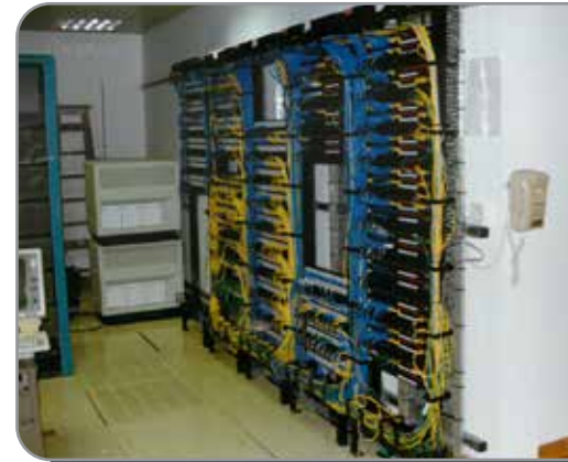
Photo above: One of our first UTP patching frames, in the heart of the City of London
